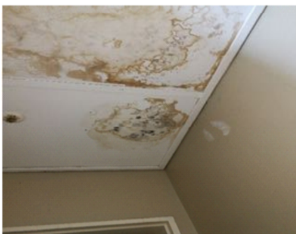
Ceiling damaged from leaking roof
