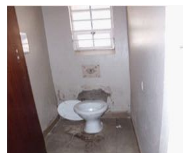
Broken Toilet in OT Department
