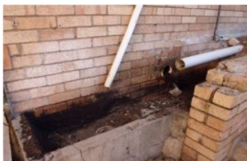
Broken drainage pipes and blocked drain at the main kitchen
