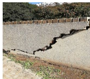
Cracked wall outside OT workshop
