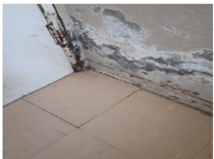
Rising damp on walls
