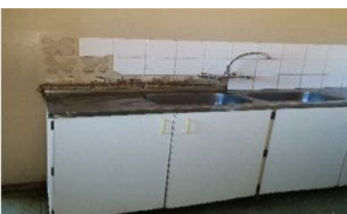
Broken tap, blocked drain and tiles peeling from the wall in the OT department
